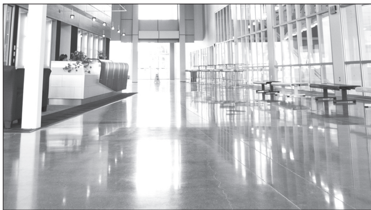
The $65.5 million Athletics and Events Center had cracked floors when it first opened its doors to the Ithaca College community in 2011.
