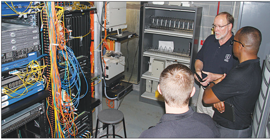
Clockwise from top, Mike Dixon, Keith McIntosh and William Weeks discuss the college's wireless infrastructure in a server room in the Roy H. Park School of Communications. COURTESY OF MATT GORNEY
