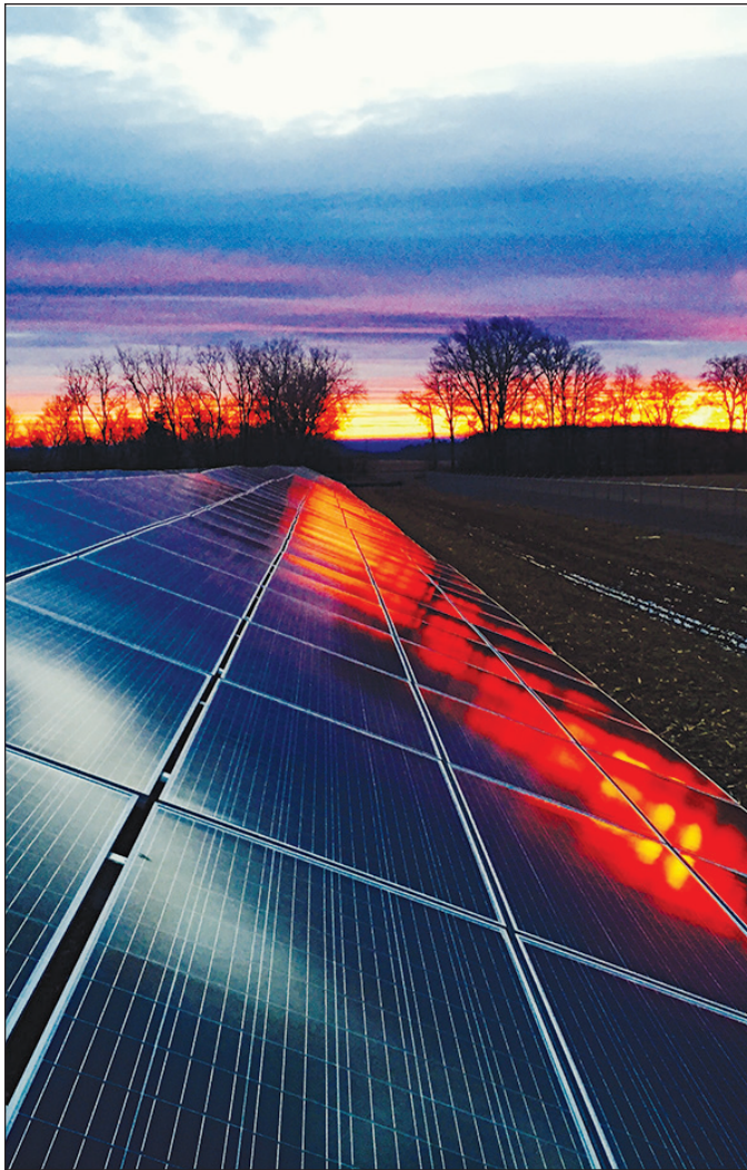
The 9,000-panel solar array is currently under construction in Seneca, New York, about 40 miles away from campus, and will cover 10 percent of the college's energy needs.
