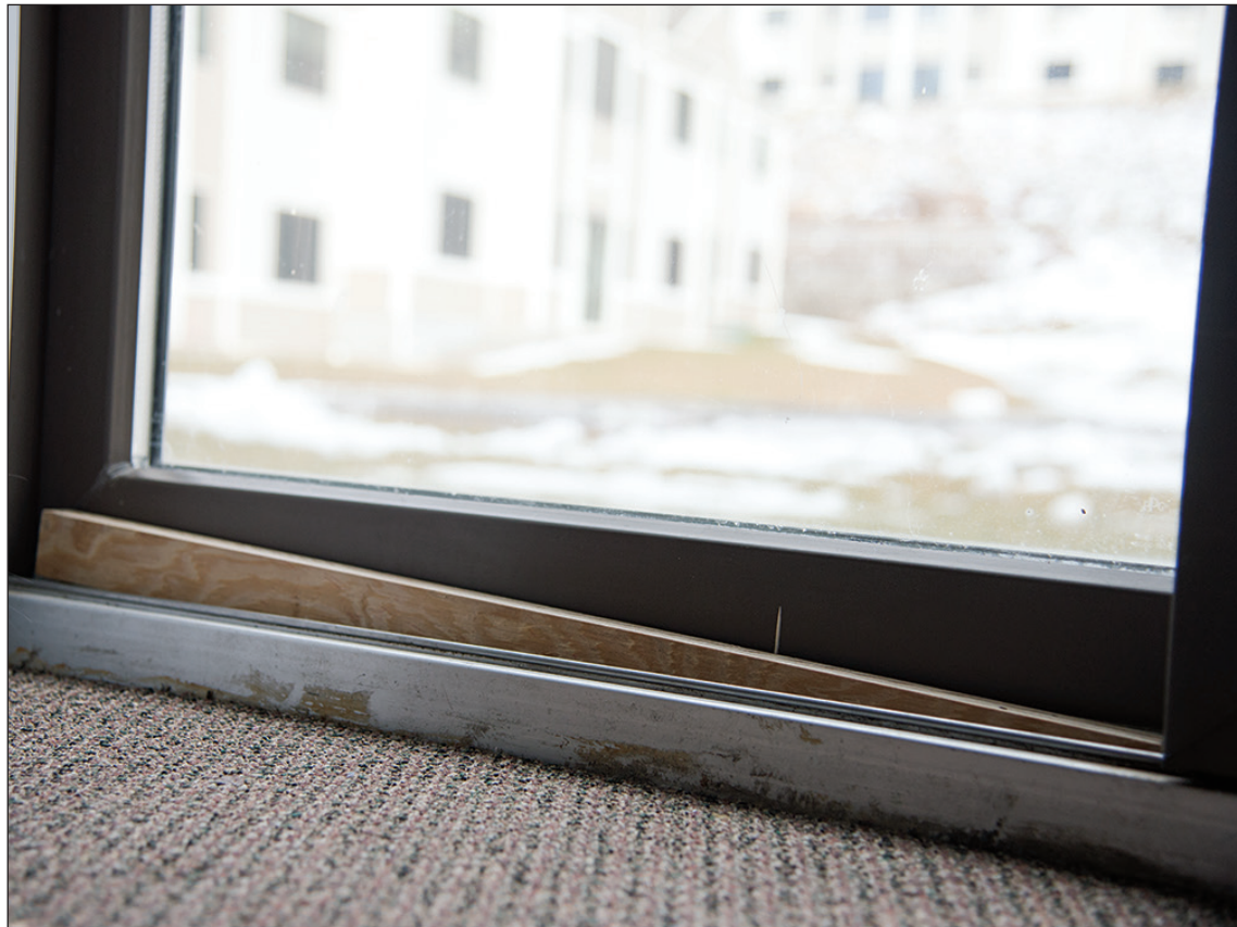
Students have been offered the option to pick up wooden blocks to be inserted inside the track of their sliding doors. The wooden block forces the door into the closed position without requiring expensive modifications.
