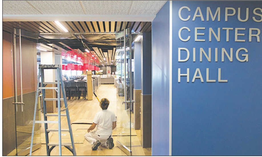
The final touches are added to the Campus Center Dining Hall on Aug. 22. Campus Center is one of the facilities that was updated over the summer on the campus.
