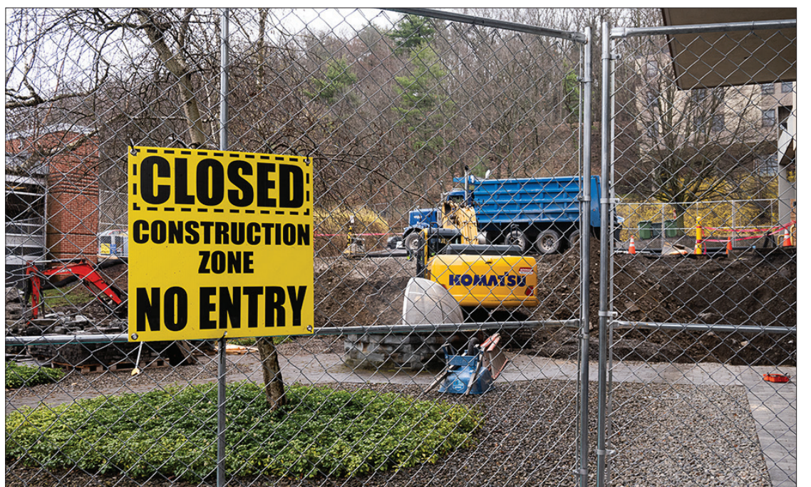
Construction for the Terrace Elevator Connector project started April 1. The southeast stairwell of the dining hall will be closed and students in Terraces will get their mail in the Towers mail lockers.
