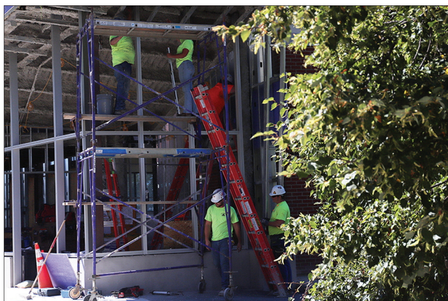
Terraces Dining Hall construction started April 1 and was scheduled to be completed during summer 2024. Now, the construction will tentatively end in September.
