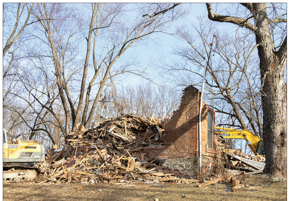
The brick building owned by Ithaca College located at 929 Danby Road was deconstructed beginning Jan. 9 after receiving a demolition permit Jan. 8.
